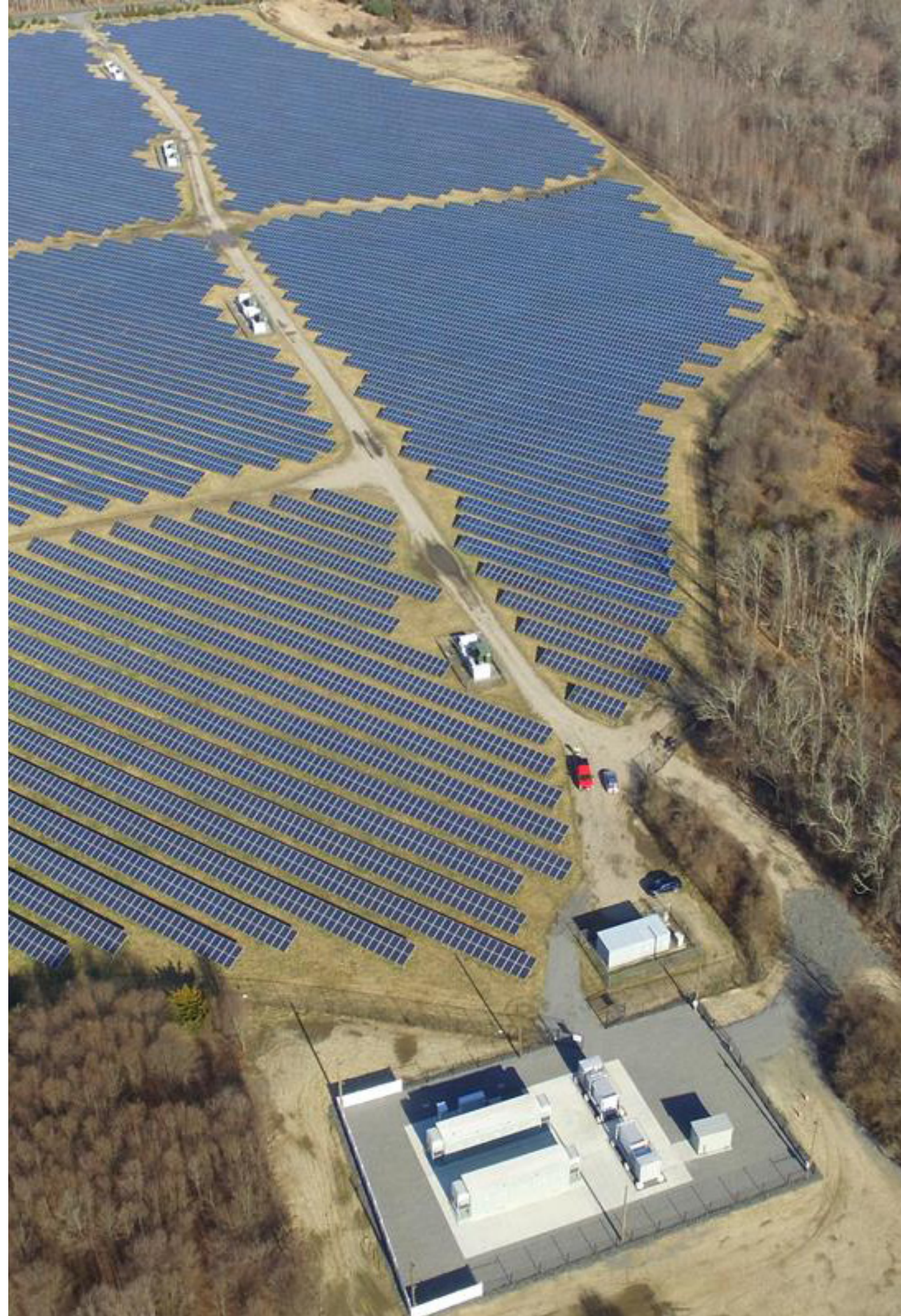
Howell, NJ, U.S., 7 MW \ 7 MWh
