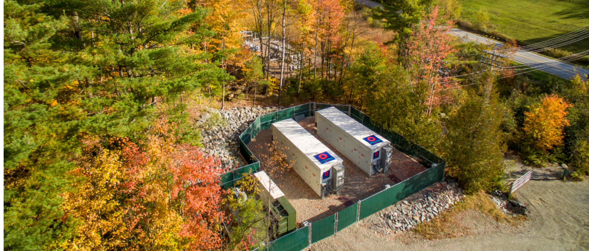
Hinesburg, VT, USA, 2 MW / 5 MWh
